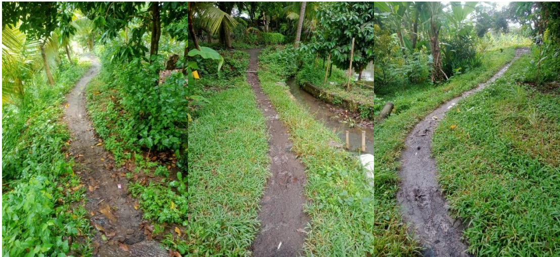
Figure 1. Condition of Existing Road Connecting Jagaraga Village
